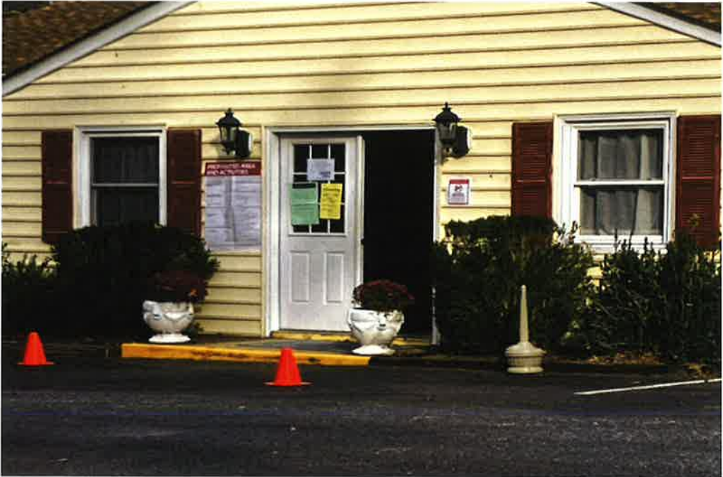
Above: New Kent- Providence Forge. No sign to reflect curbside voting or accessible entry with curb-cut.
