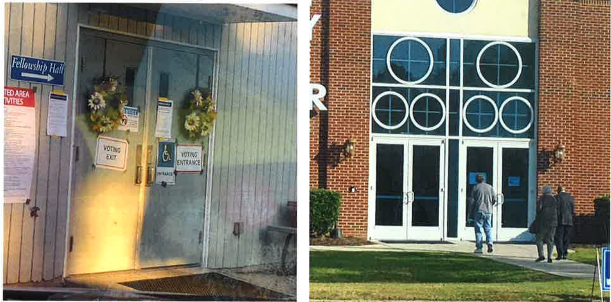
Above: Inaccessible doors in Chesapeake, VA.
